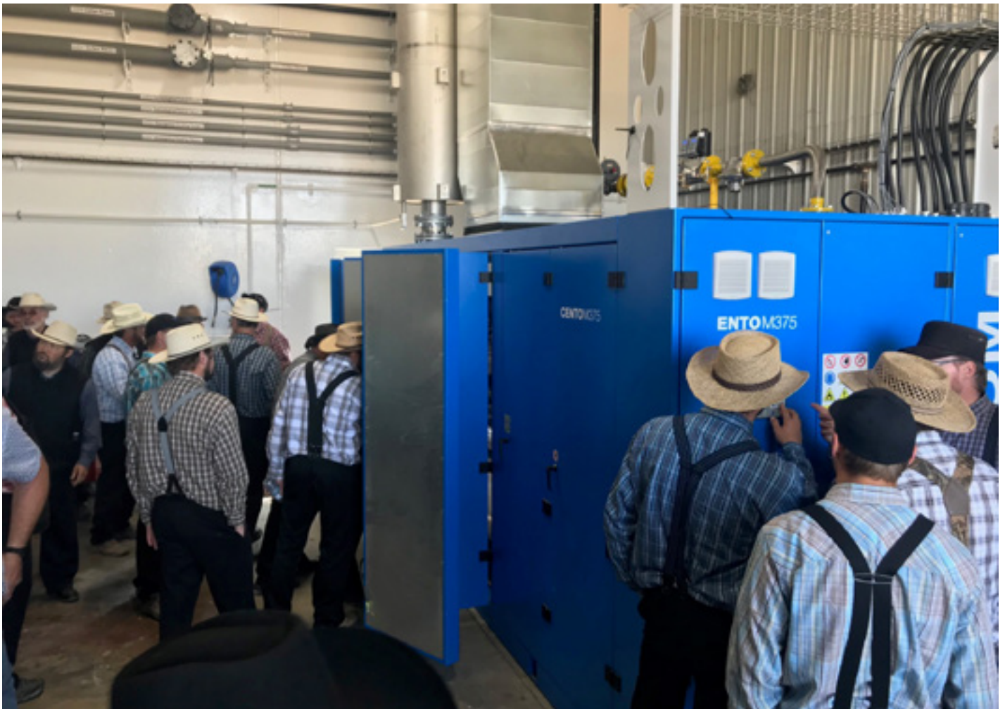
This combined heat and power unit, installed at a farm near Bashaw, Alberta – about 150 kilometres southeast of Edmonton – is one example of Canadian pork sector energy innovation, but it comes with a large capital cost.
