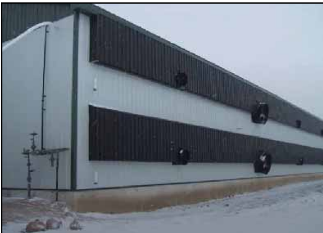
Example of a barn with a transpired solar collector, also called a solar wall
