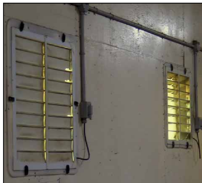
Shutters on fans are used as backdraft devices to prevent the fan from acting as an air intake
