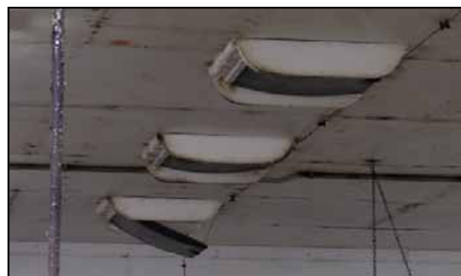
These air inlets should be adjusted and calibrated to introduce air uniformly
