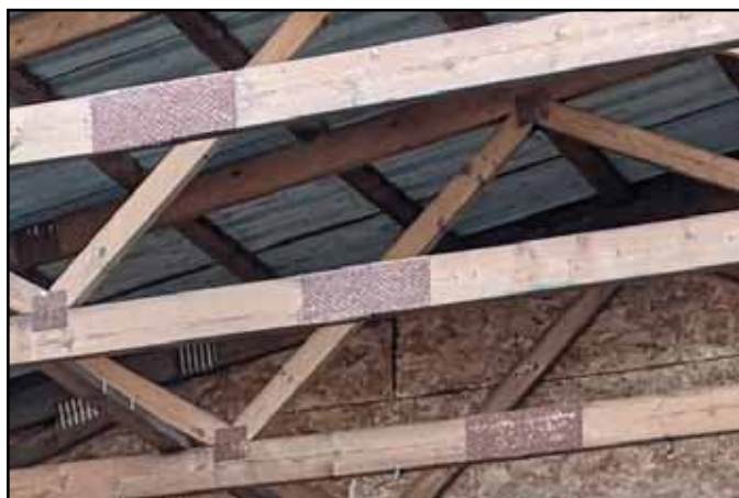
Ensure there is no corrosion on brackets, truss plates, pins and rafters
