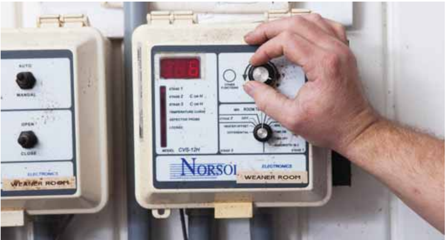
Automatic ventilation systems with ventilation curves can optimize the barn environment and reduce the need for antimicrobials.
