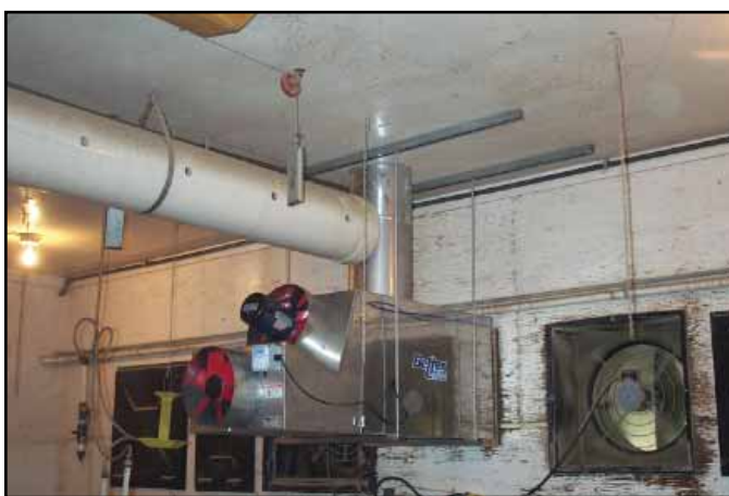
An air-to-air heat exchanger installed at Prairie Swine Centre
