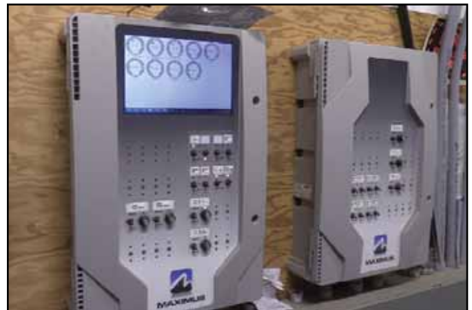
Centralized controller system for an entire barn
