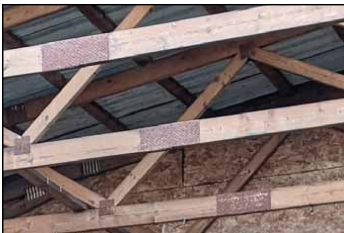
Ensure there is no corrosion on brackets, truss plates, pins and rafters
